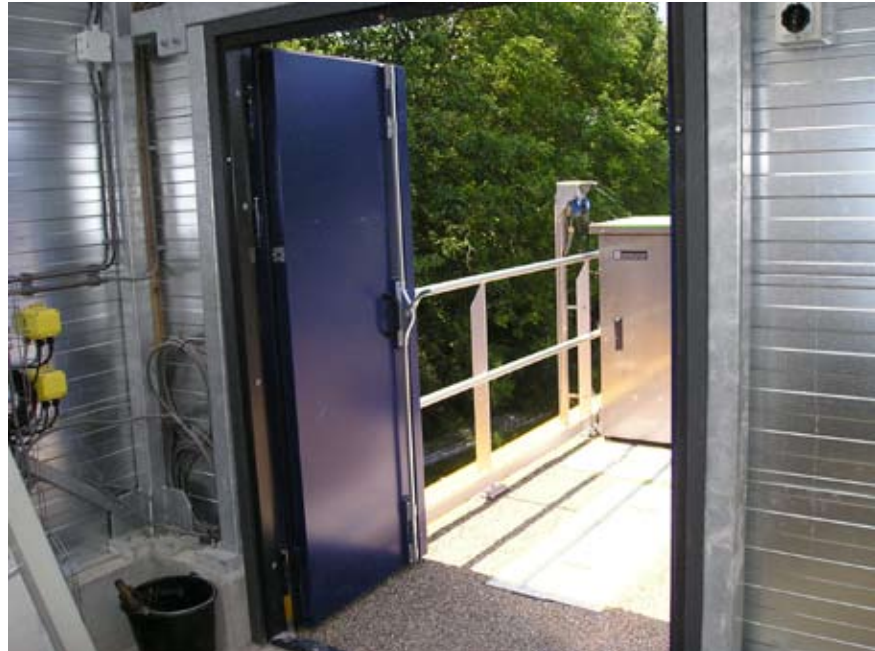
MN 41 Sewage Treatment Overvecht
